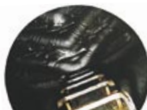
Photos showing vertical movement of cooling water tubes at
